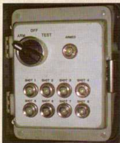
The onboard RF pyrotechnic system hidden within the prop seaplane. The onboard pyrotechnic system is linked to the attraction's overall control system by an early implementation of the wireless Ethernet systems popular today.
