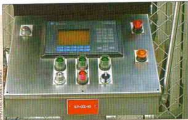
The seaplane launchers' console outside the secure area backstage. Like the main console, it subscribes to a standard labeling, appearance, and placement of operator controls. Status and diagnostics from this subsystem are forwarded to the attraction's main control system.
